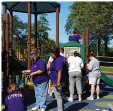
Volunteers from Kohl's Department Stores joined forces with other helpers to install new play equipment at Augusta Playground Park in the West Humboldt Park neighborhood.
