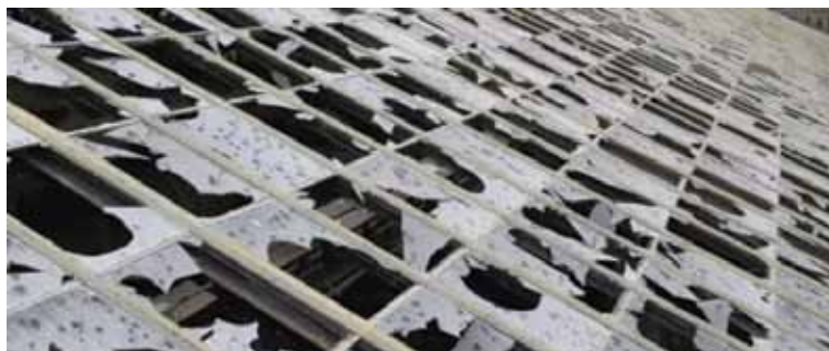
Hail caused millions of dollars of damage to Garfield Park Conservatory during a recent storm.
