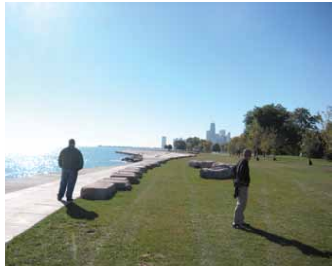
The Belmont-Diversey Revetment project, which began in April 2003, removed old crumbling limestone protection barriers from a 1,700-foot stretch along the lake and replaced them with a new multi-tiered concrete structure that can also be used as a pedestrian promenade.
